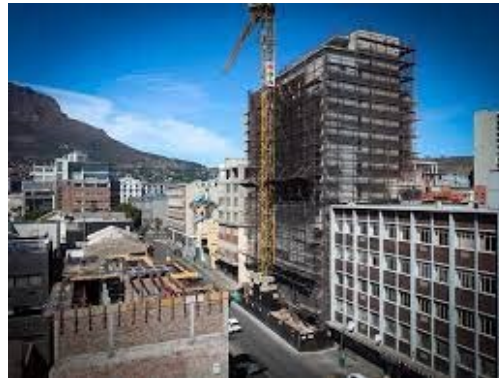
Cape Town hemp building estimated to be tallest hemp building in the world.
