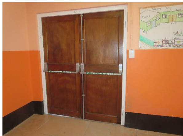
Supply and Fit Security Doors and Push Bars as per Fire Requirements for Nomaxibiso ECD Facility (City of Cape Town)
